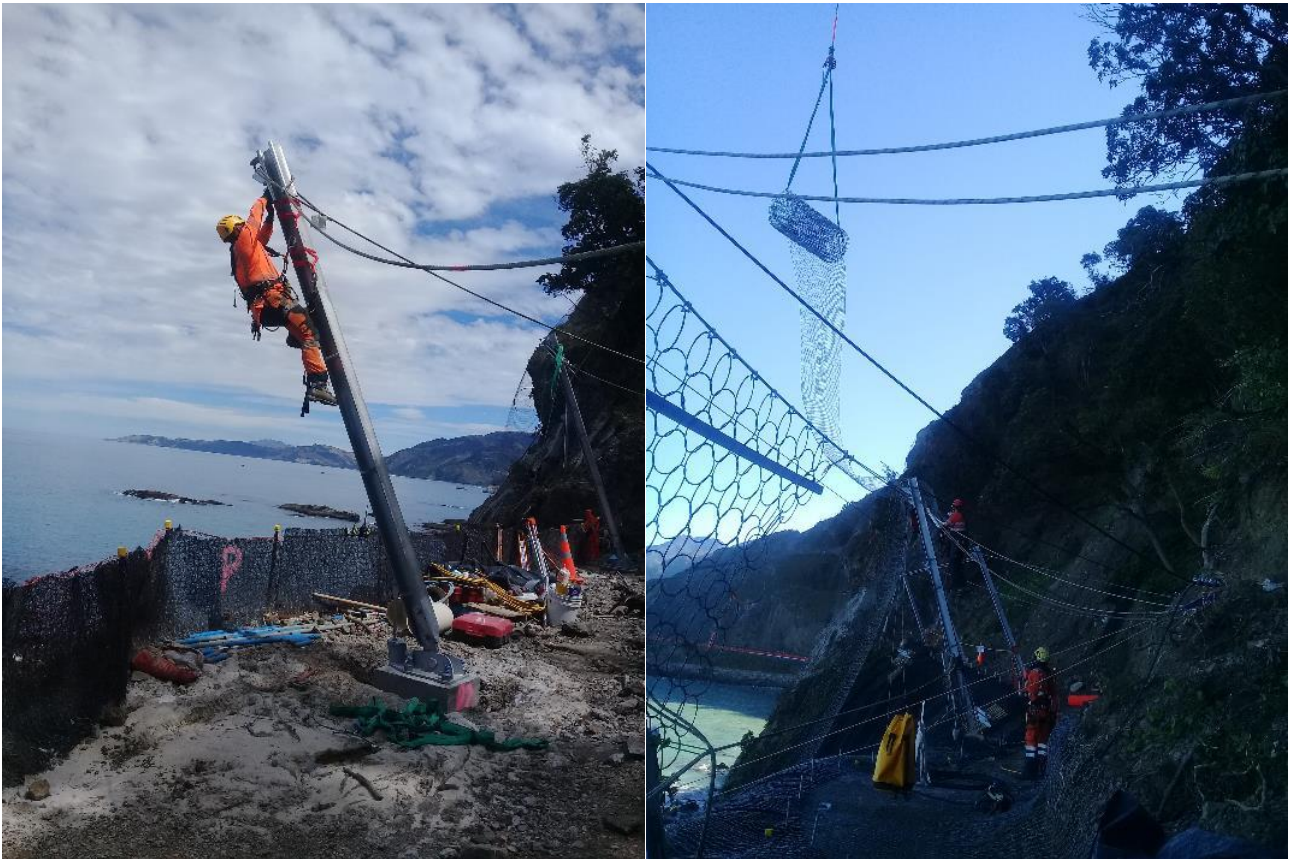
Figure 2 (left): Construction of shallow landslide barrier, Slip 18 south of Kaikōura, Nov. 2017. Figure 3 (right): Installing mesh by helicopter sling load, a high-risk activity, Slip 18. Heli-operations were often conducted over an open highway during short road closures to minimize disruption to the travelling public. Compression of these types of construction activities in time and space increased the risk for workers.
