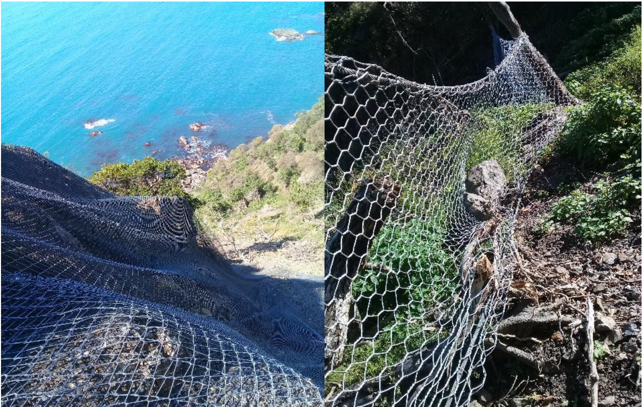
Figure 6 (left): Example of temporary rockfall mesh installed above an occupied worksite, Slips 18 & 19, south of Kaikōura. This structure contained a ~100 m 3 failure which occurred during rainfall, June 2017. Figure 7 (right): Temporary rockfall catch fence above worksite, Slip 18. This structure was impacted 4 times by rocks ~1m 3 during the course of construction of a shallow landslide barrier directly below. Photos: R. Musgrave.
