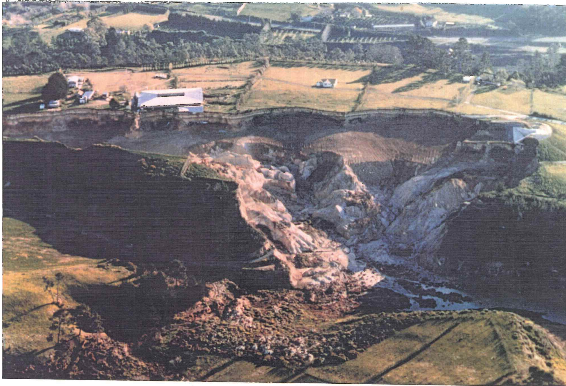
Photo 1. The Ruahihi canal failure
